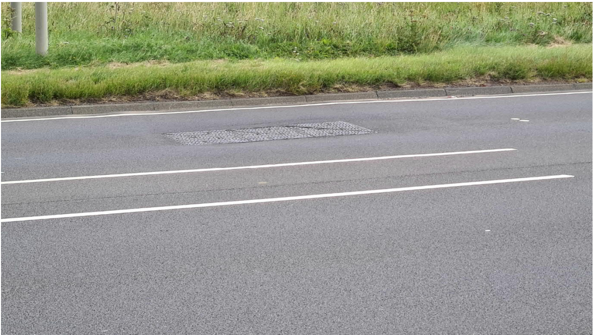
Photo 1 - Manhole on A1 capacity to be checked
