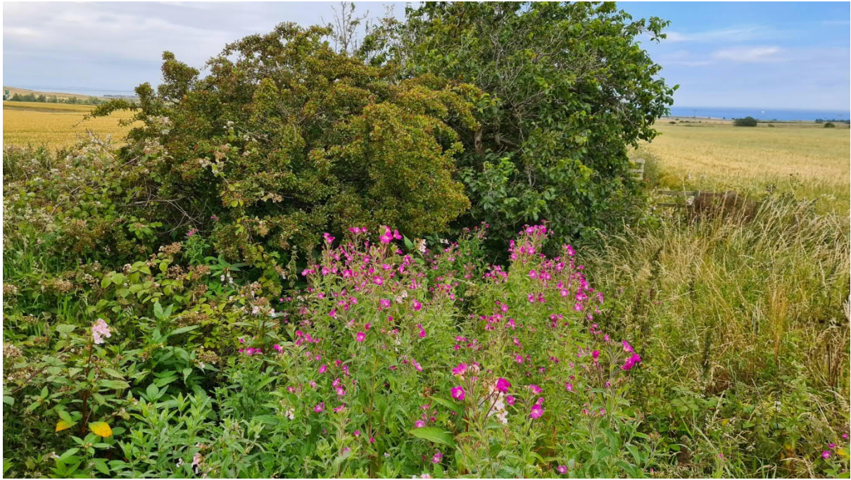
Photo 13 – Overgrowth at culvert outlet
