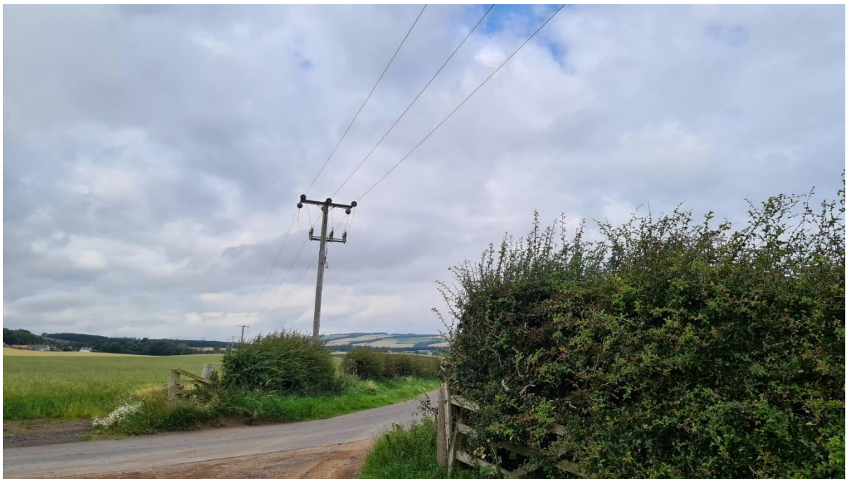
Photo 16 – Overhead lines at junction to New track
