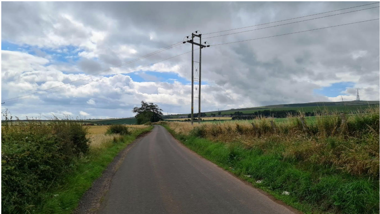
Photo 10 – Overhead lines chainage 700 Drawing 103
